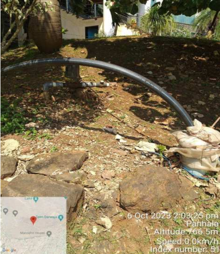
Photograph: Bore well water recharging.
