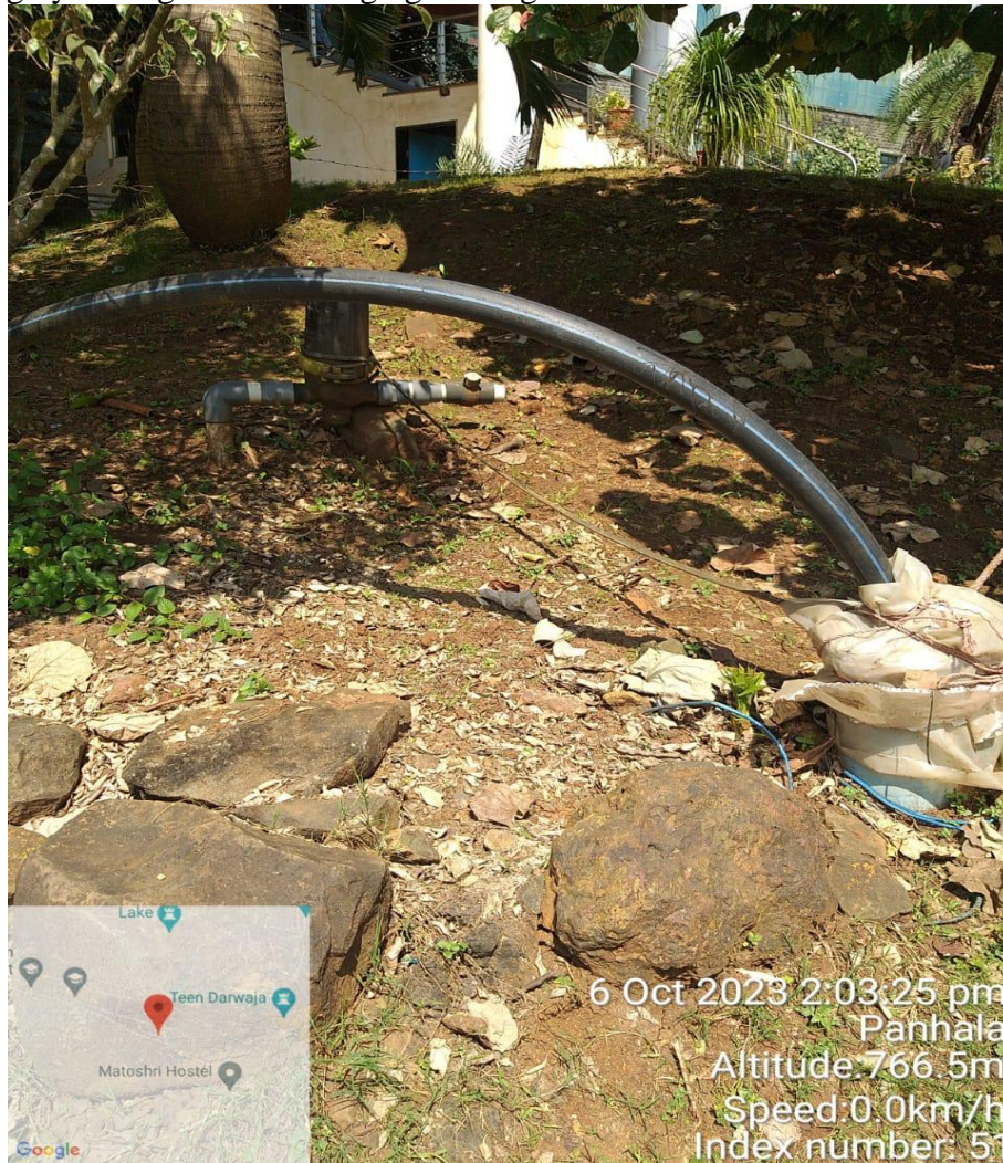
Photograph: Bore well water recharging.
